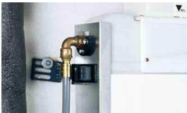
Potable water installation
